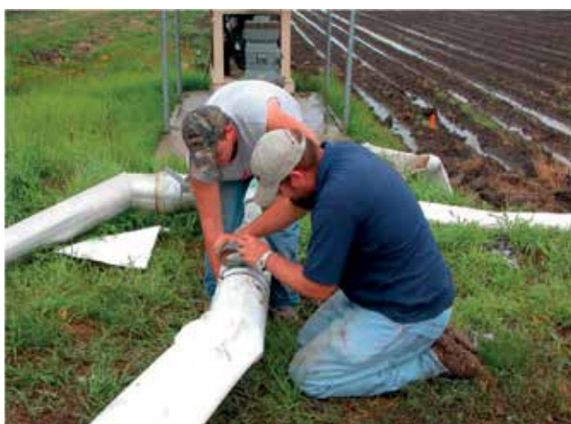
Figure 2. Connecting plastic tubing to well pipe with zip ties and duct tape.
