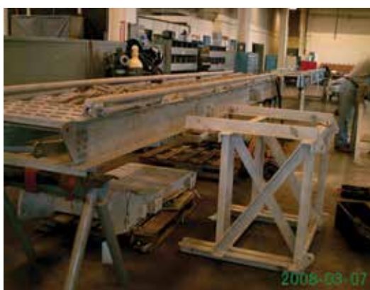
Figure 1. ACCOM ladder on work stands before intervention. The ladders are being disassembled for repair.
