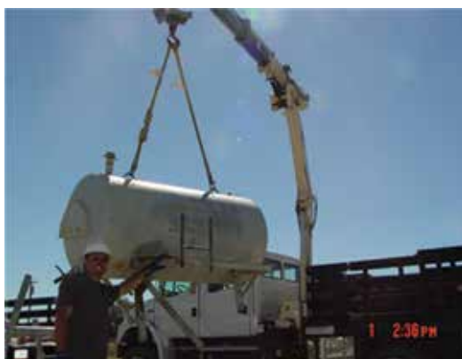
Figure 17. After intervention, truck mounted knuckle boom crane is used in operations where other material handling equipment has not been capable of performing the waste removal.
