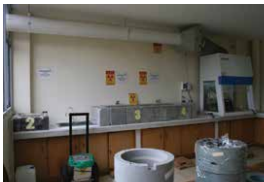
Figure 14. Concrete shielding in decay room.
