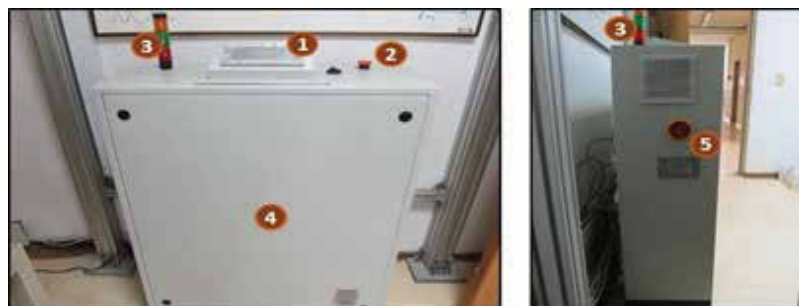
Figure 22. Positioning system: 1. HMI; 2. Emergency stop; 3. System status; 4. Electronic components; 5. Power control.
