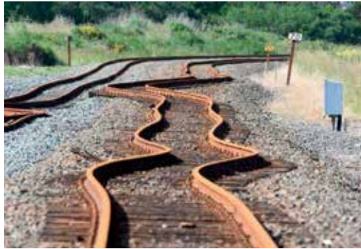
Figure 5. Twisted railroad tracks, an example of structural damages due to SH displacement of Love surface waves in the aftermath of an earthquake.
