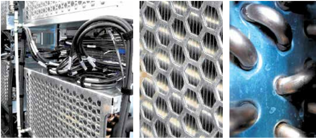
Fig. 2. Water-cooling in rack.
