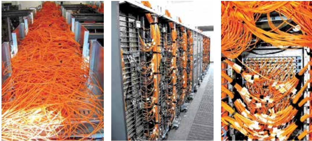
Fig. 4. Networks, cabling, switches.
