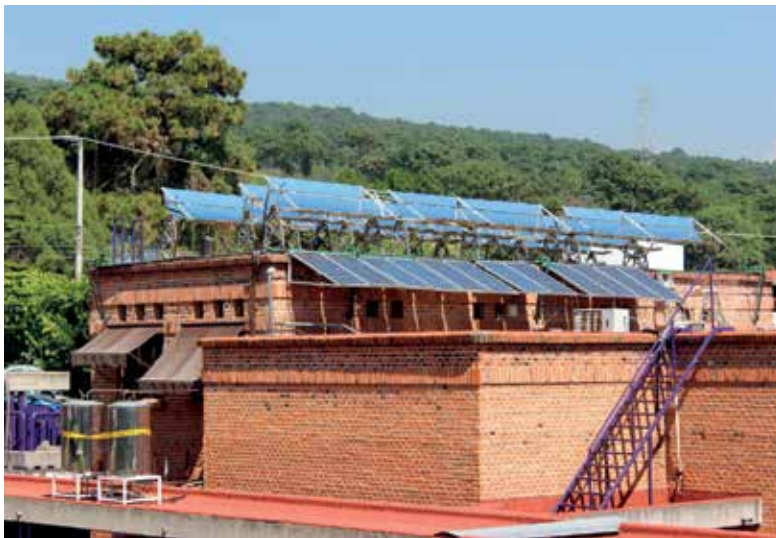
Figure 2. Photograph of the thermal and photovoltaic solar systems on the building roof.
