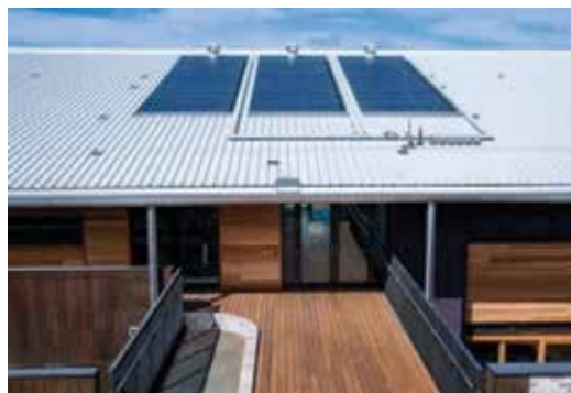
Figure 2. Air-based PVT collectors implemented in a net-zero energy office building.
