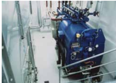
Adsorption chiller installed in the University hospital in Freiburg
