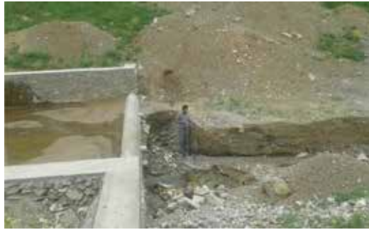
Figure 2. Misconducting of a check dam on a water way.
