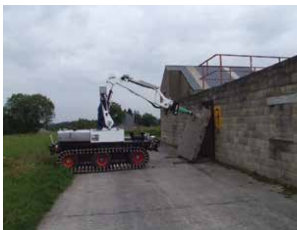
Figure 16. The LUGV uses its jackhammer to breach through a concrete plate (Source: ICARUS).
