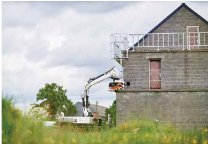
Figure 12. ICARUS large unmanned ground vehicle deploying the small unmanned ground vehicle on the top of a building (source: ICARUS).
