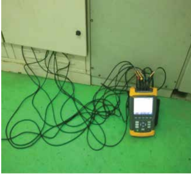
Plate 2. Monitoring equipment for PQ data collection at a substation with fluke 435.
