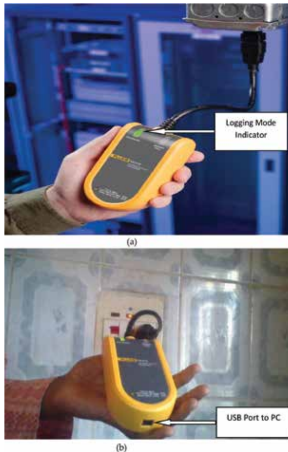
Plate 1. Voltage quality recorder (VR1710) logging data. (sources: (a) installation manual of fluke VR1710 (b) at a residential power outlet in Bauchi).
