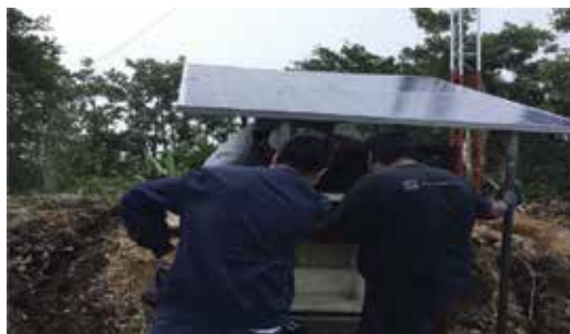
Figure 10. Installation of a mini solar PV system for telecommunications purposes, a rural community in Oaxaca Mexico.
