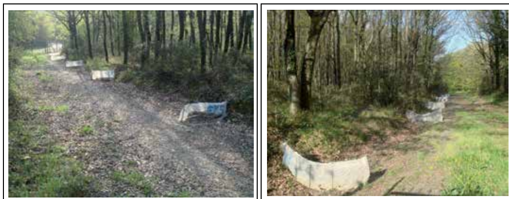
Fig. 4. Sediment traps on forest road and collected sediments on sediment traps at Belgrad Forest-Istanbul, Turkey (Kartaloglu, 2011).
