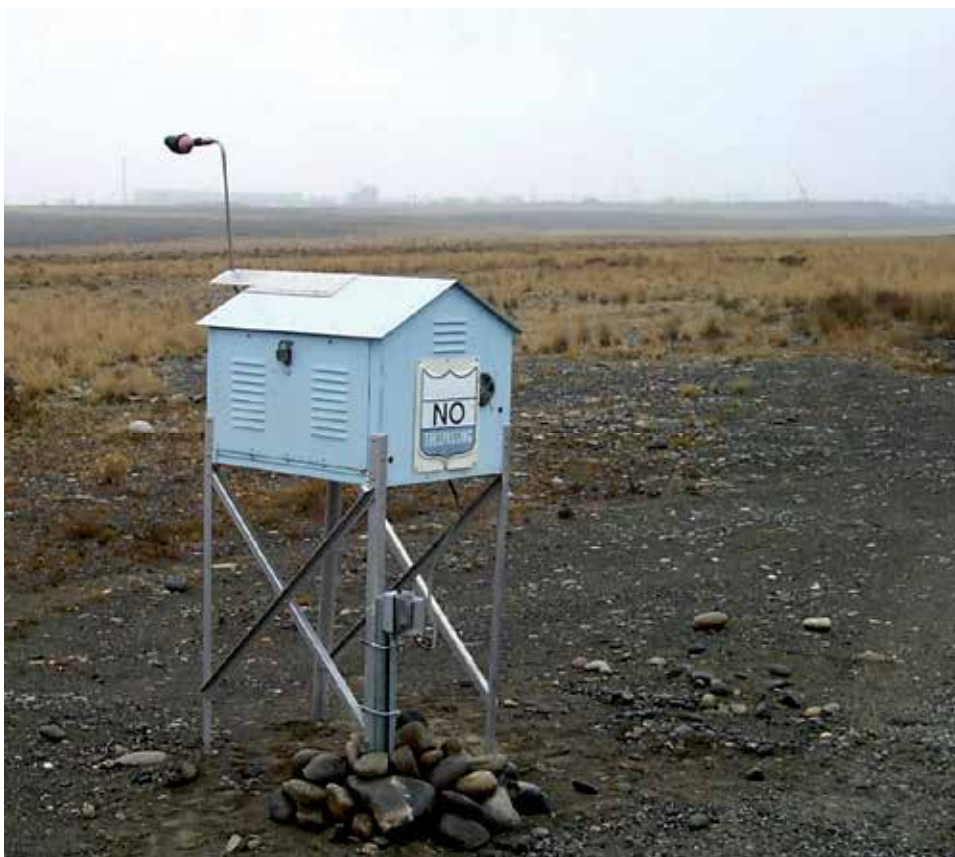
Fig. 5. Environmental air monitoring station
