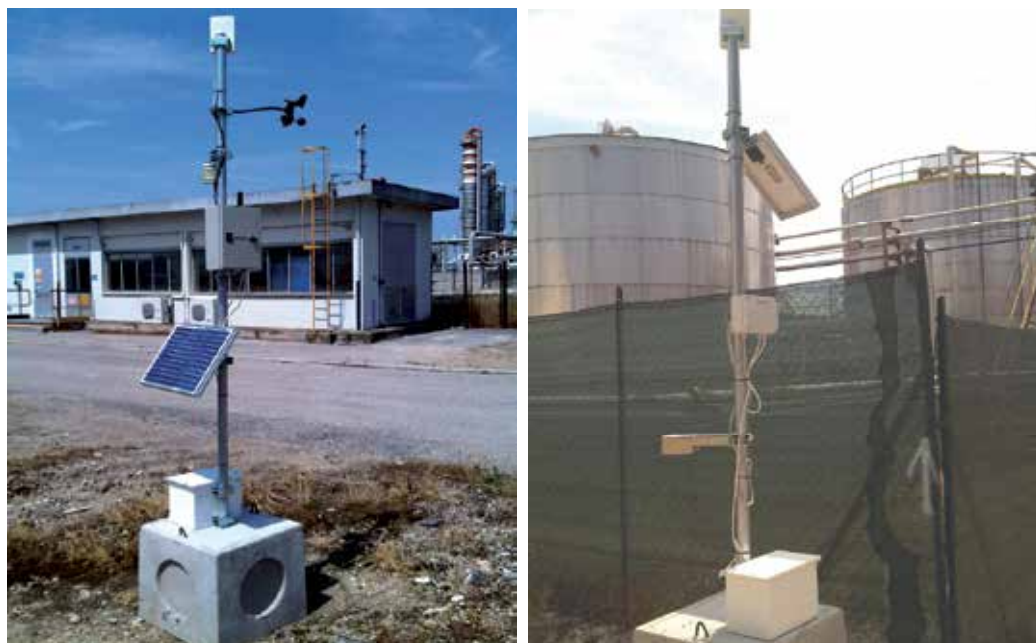
Fig. 6. SN (left) and EN (right) units installed in proximity of the pipeline and of the chemical plant
