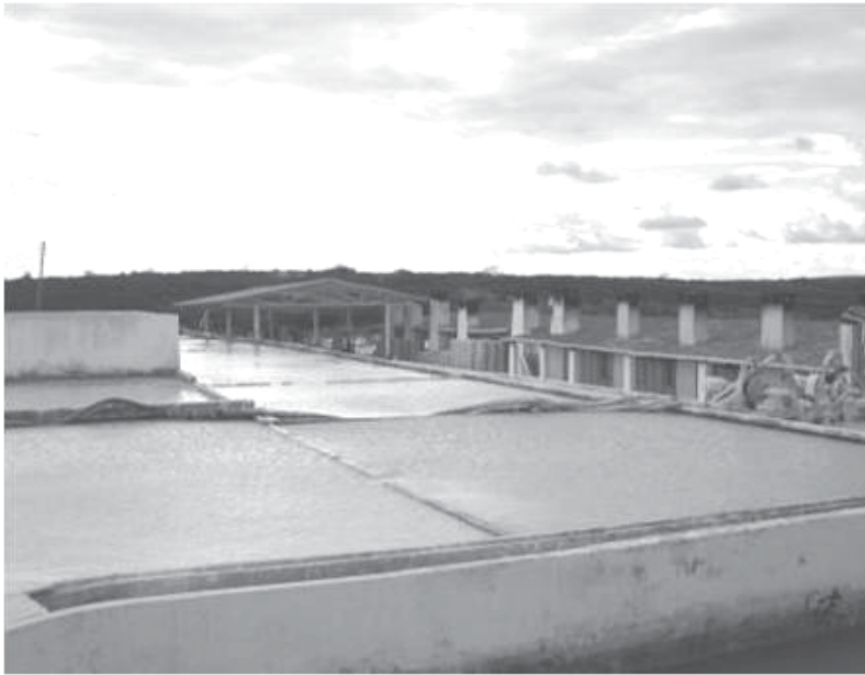
Fig. 8. Sedimentation tank used in the second step of kaolin processing
