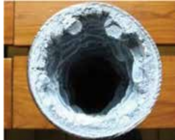
Figure 4. Heavy build-up of deposition on heat exchanger piping [24][23].
