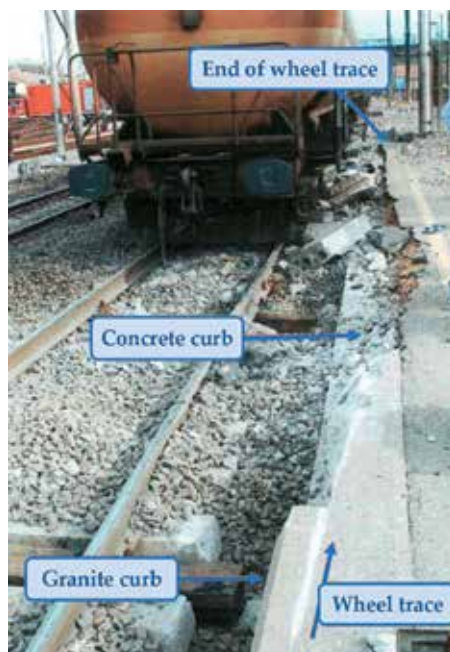
Figure 6. Concrete sidewalk damaged by the right wheel of the front wheelset of the first bogie of carriage no. 1 and starting point of the carriage overturning.
