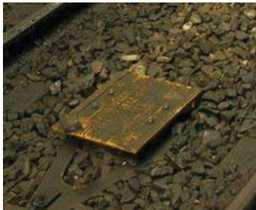
Figure 3. Example of balise mounted on the track.
