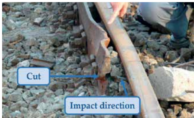
Figure 19. Check rail opposite to the wing rail photographed during the investigations on the accident site conditions.
