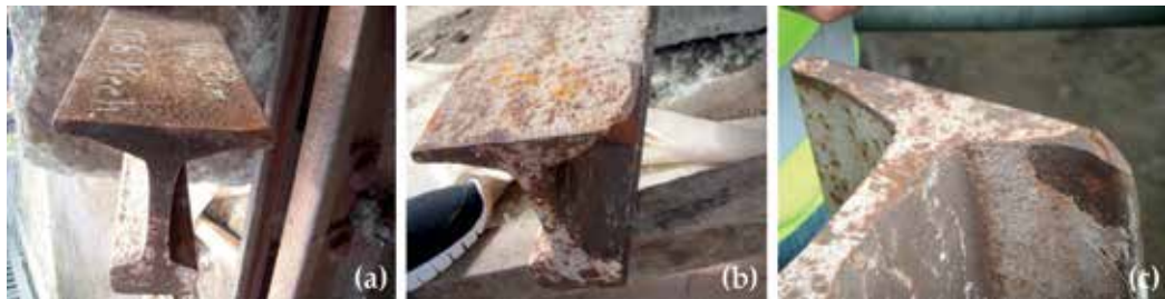
Figure 16. Track reference stake no. 24 photographed after its extraction from the track ballast. (a) In the foreground: flange of the track reference stake with damaged edge; in the background: view of the concrete plinth; and (b) and (c) details of the damaged edge.
