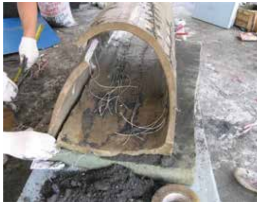
Figure 13. The fracture of the liner (right tunnel) in case 1.
