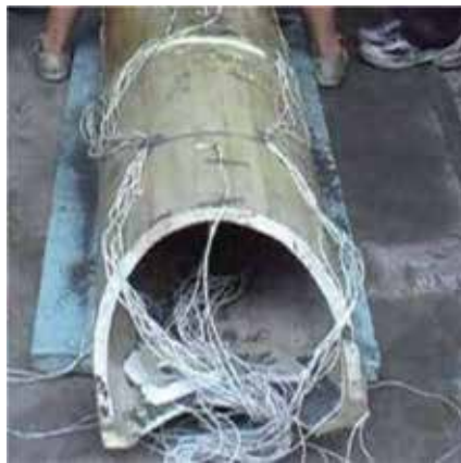
Figure 14. The fracture of the liner with soft isolation layer (right tunnel) in case 2.
