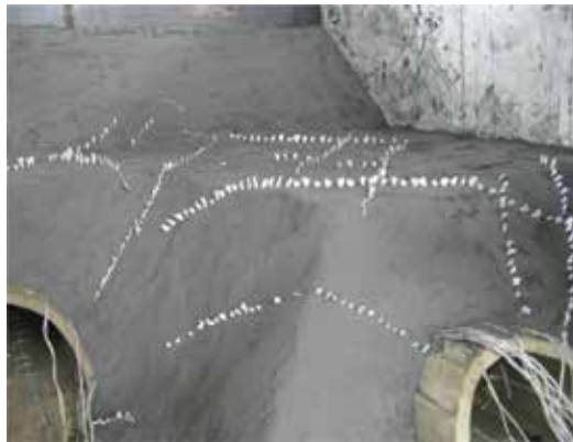
Figure 11. The distribution of ground cracks.
