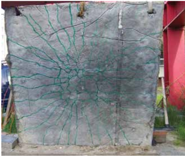
Figure 6. Cracks on the bottom surface of the slab.
