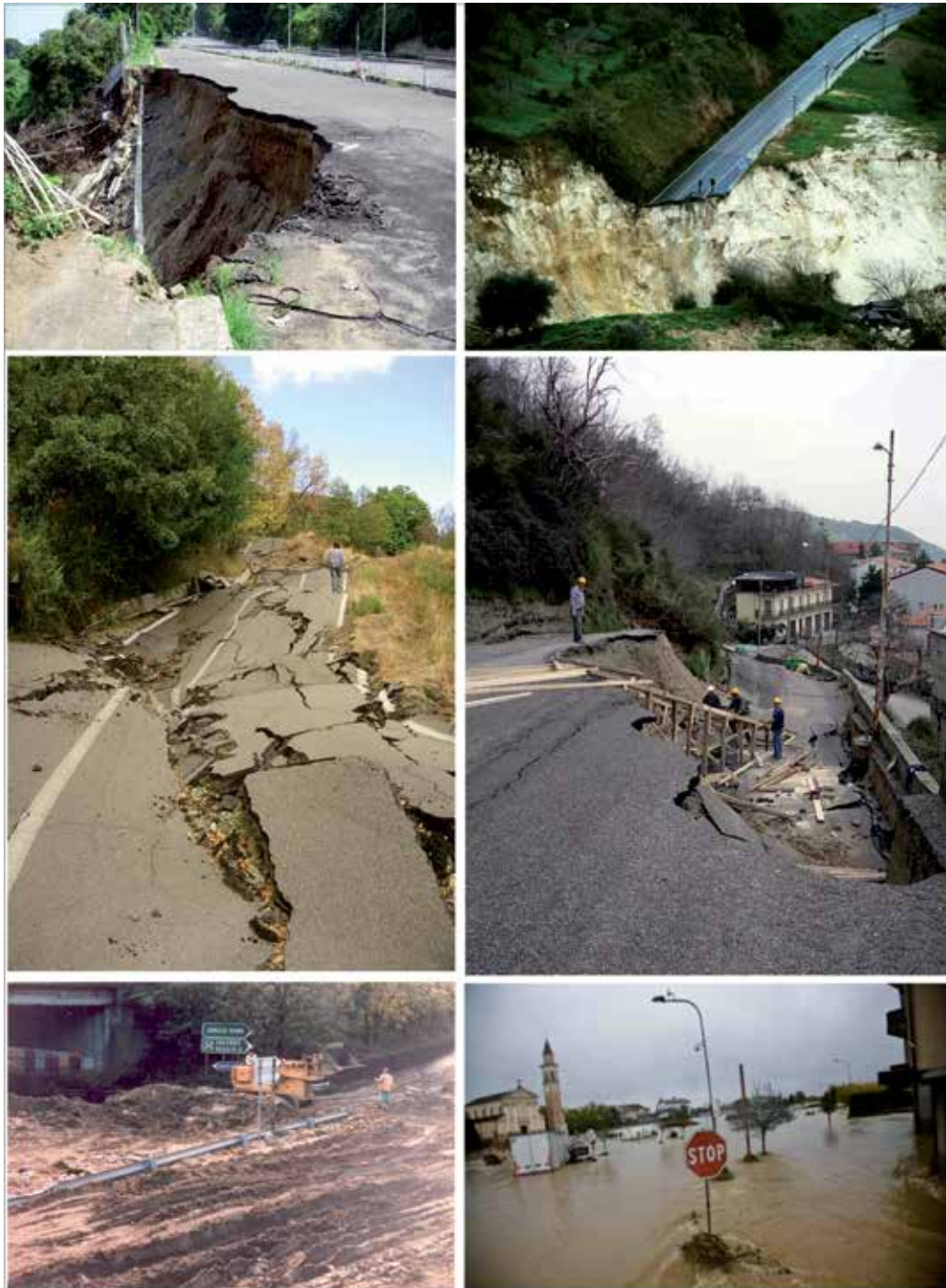
Fig. 1. Damage caused to roads by landslides and floods in Calabria.
