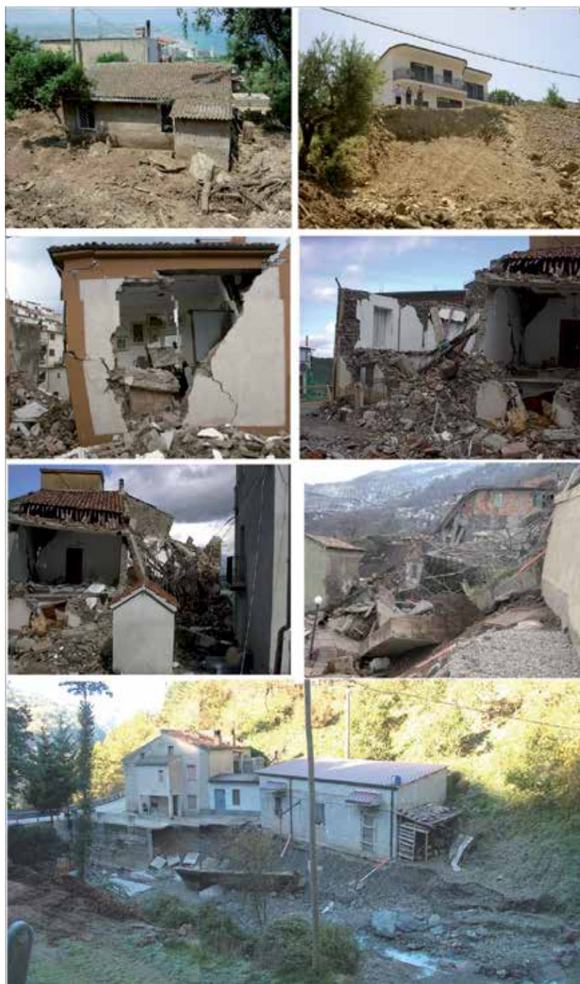
Fig. 2. Damage to houses caused by landslides and floods in Calabria.
