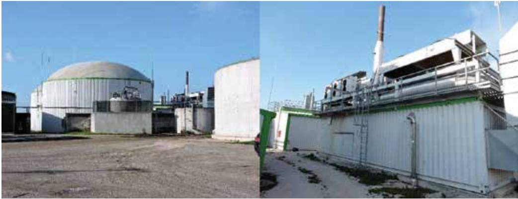
Figure 3. Power generation plant (1 Mw) fed with wet olive husks and wastewaters from the olive oil extraction. Biogas is generated in the digester (right) and stored (left), then converted into electricity. Installation Friel Ionica Srl - BTM Srl spinoff of the University of Pisa, located in Manduria (Taranto, Italy) (Source: Marco Nuti).
