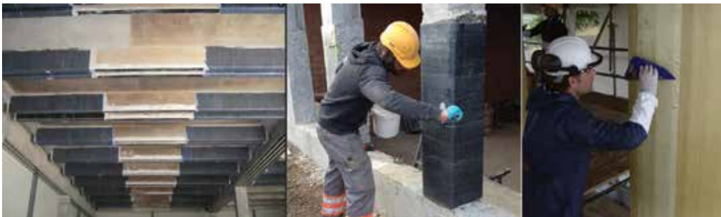
Figure 14. Strengthening of existing concrete structural members using unidirectional carbon and aramid sheets [98].
