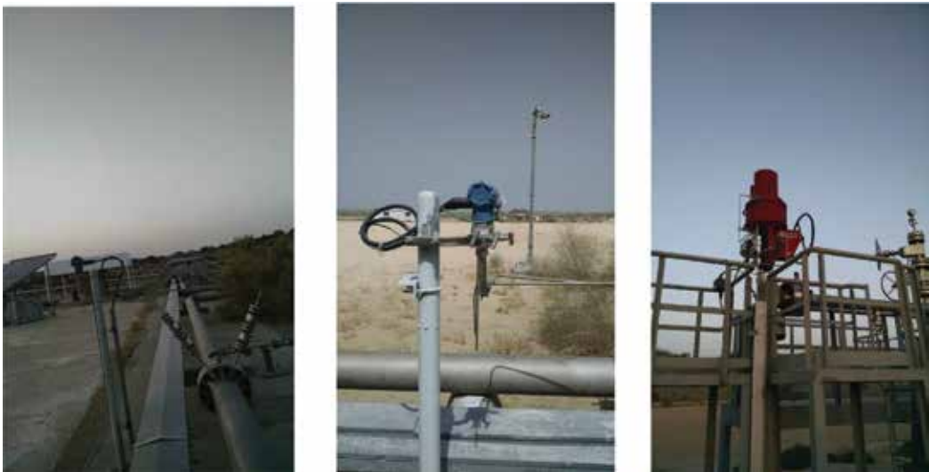
Figure 11. Flow control valve, pressure gauges, and process flow lines.
