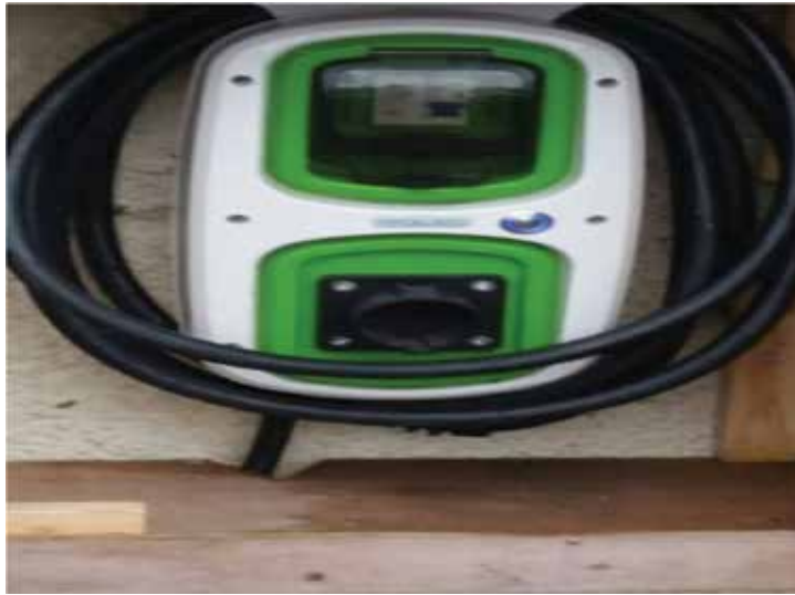
Figure 14. Domestic electrical vehicle charger.
