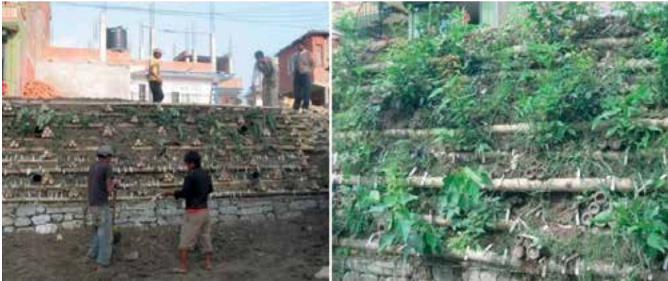
Figure 7. The vegetated bamboo crib wall just after construction (November 2006) and after 1 year of construction (Kusunti, Lalitpur, November 2007) [26].
