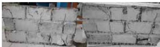
Figure 6. Collapse of concrete block wall sample after being tested [3].
