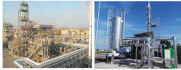
Figure 6. Chemical plant and hydrogen sulfide tank.
