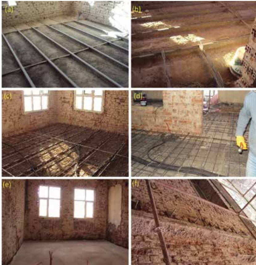
Figure 6. Retrofitting of jack arched slabs: (a) removing top layers of the slab, (b) welding of shear rebar over I-profile beam, (c) steel tie, (d) connections of stainless steel ties between the masonry walls, (e) anchorage of stainless steel, and (f) topping concrete application on slab.
