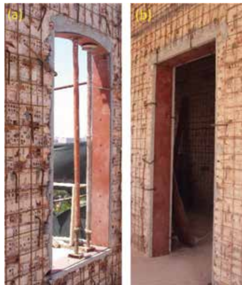
Figure 7. Retrofitting of door and window gaps using steel plates (a and b).
