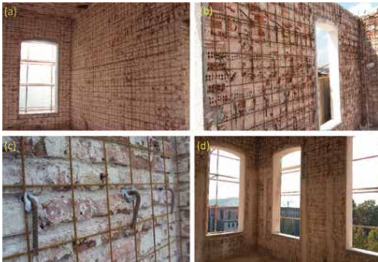
Figure 5. Retrofitting of the internal walls after plaster removal: (a–c) rebar grid technique and (d) application of thick plaster.
