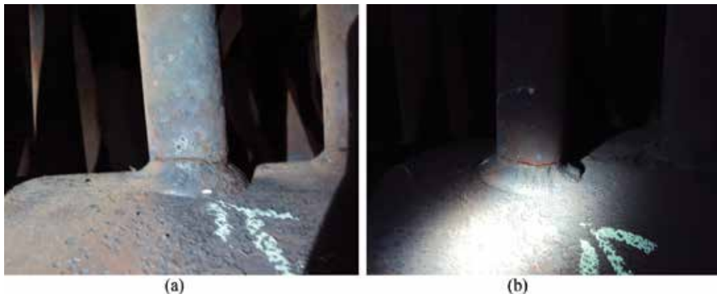
Figure 2. Appearance of Row 3 tube failures, (a) Tube 8 and (b) Tube 9.
