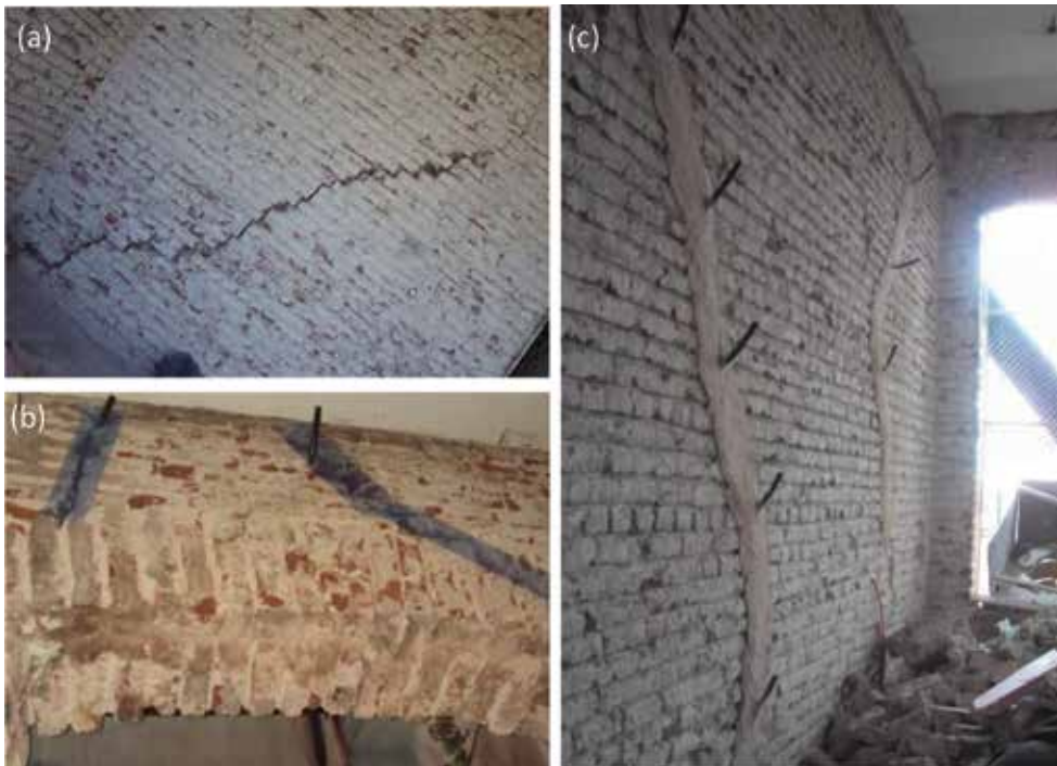
Figure 3. Injection application in the walls after plaster removal: (a) structural cracks, (b) preparation of wall surface for injection, and (c) injection application by manual technique.
