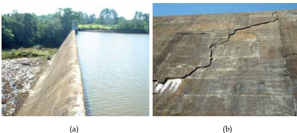
Fig. 8. (a) Overview of the spillway of the dam. (b) Detail of the displacement of the surface caused by hydraulic abrasive processes.
