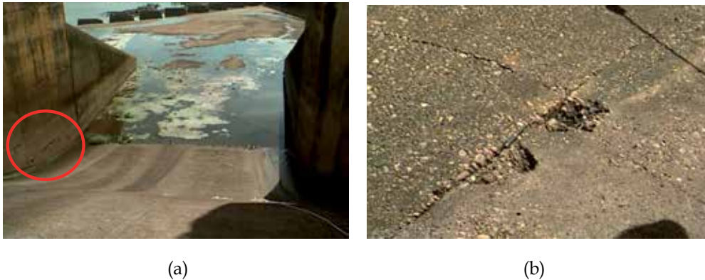
Fig. 2. (a) Spillway dam presented deterioration by abrasion. (b) Defects in the concrete structure caused by abrasive process
