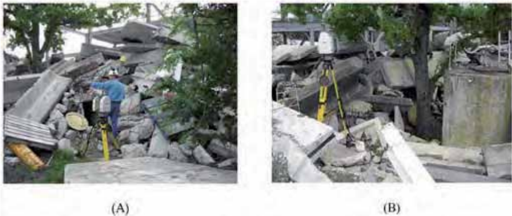
Fig. 13. (A) Setting up a scan of the rubble pile. Scan locations must be carefully chosen to obtain sufficient scene data to capture the existing conditions and enable tie in to prior scans using pre-positioned targets. (B) Since the laser scanner is a line-of-sight device, obtaining sufficient information for a disordered scene such as the rubble pile requires numerous scan locations throughout the environment.
