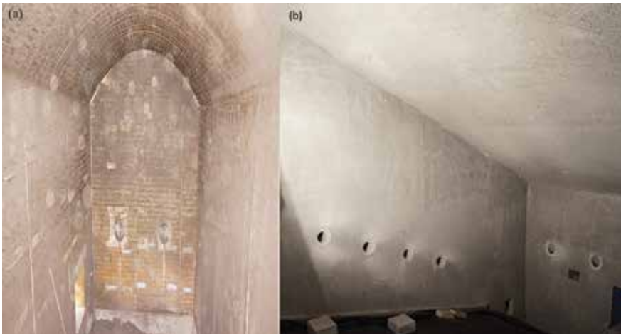
Figure 2. Biofuel boiler lining made of (a) fired bricks and (b) castables.
