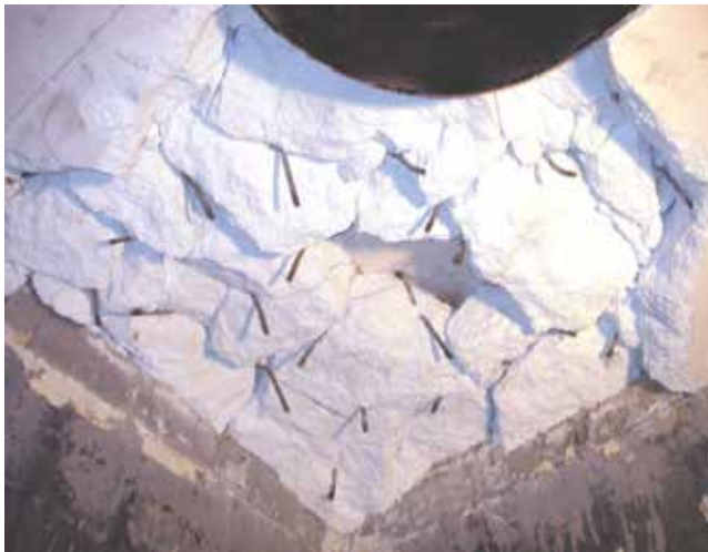
Figure 12. The part of the combustion zone structure in the heating unit used in oil refineries damaged by explosive spalling (metal anchors can be seen on the photograph) [29].
