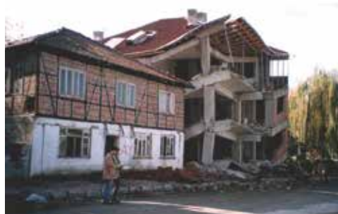
Figure 1. Different damaged conditions of traditional wooden and reinforced concrete buildings after the 1999 Duzce earthquake. Image taken from [6].
