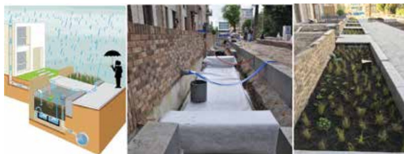
Figure 4. Left to right: Schematic of the green stream system, under construction and on the day of completion.
