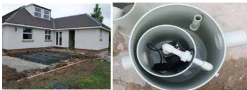
Figure 1. Left: Skeletanks® in place and connected together. Right: lightweight pump chamber.
