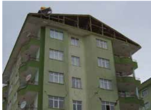
Figure 16. Failure of gable walls on top of the building during the Van earthquake.
