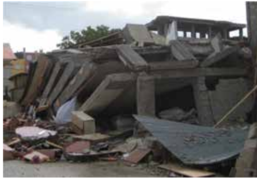
Figure 15. Failure of a building due to strong beam–weak column effect during the Van earthquake.
