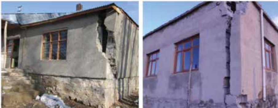
Figure 20. Corner damage of briquette masonry buildings [42].
