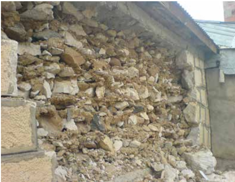
Figure 23. Disintegration in stone masonry buildings [28].
