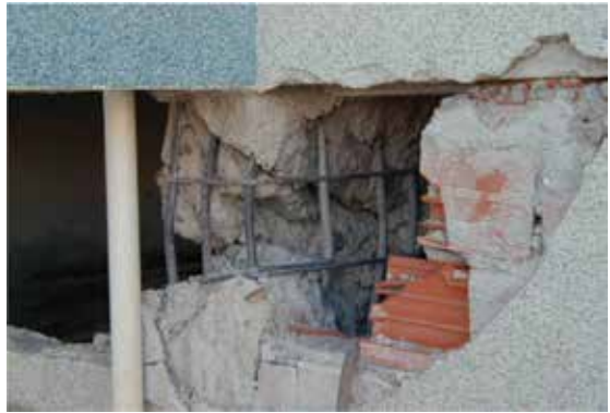
Figure 13. Short column damages during the 2003 Bingöl earthquake.
