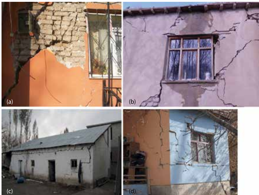
Figure 22. Diagonal shear (a-b), horizontal (c) and stepped (d) failures wall [42].
