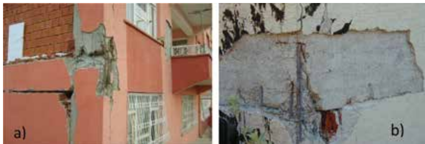
Figure 12. Damaged structure due to inadequate spacing between shear reinforcements during (a) Van earthquake and (b) Bingöl earthquake.
