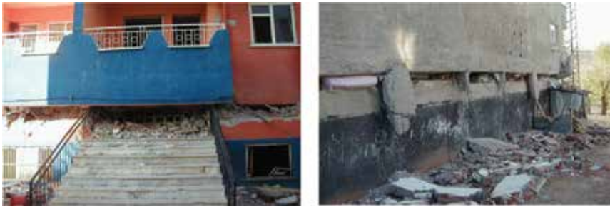
Figure 11. Weak storey mechanism during the Bingöl earthquake.
