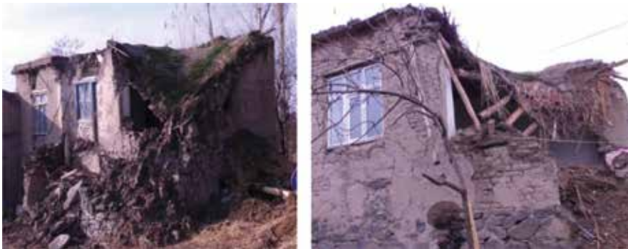
Figure 19. Damage to adobe structures due to heavy earthen roof during the Van earthquake [42].
