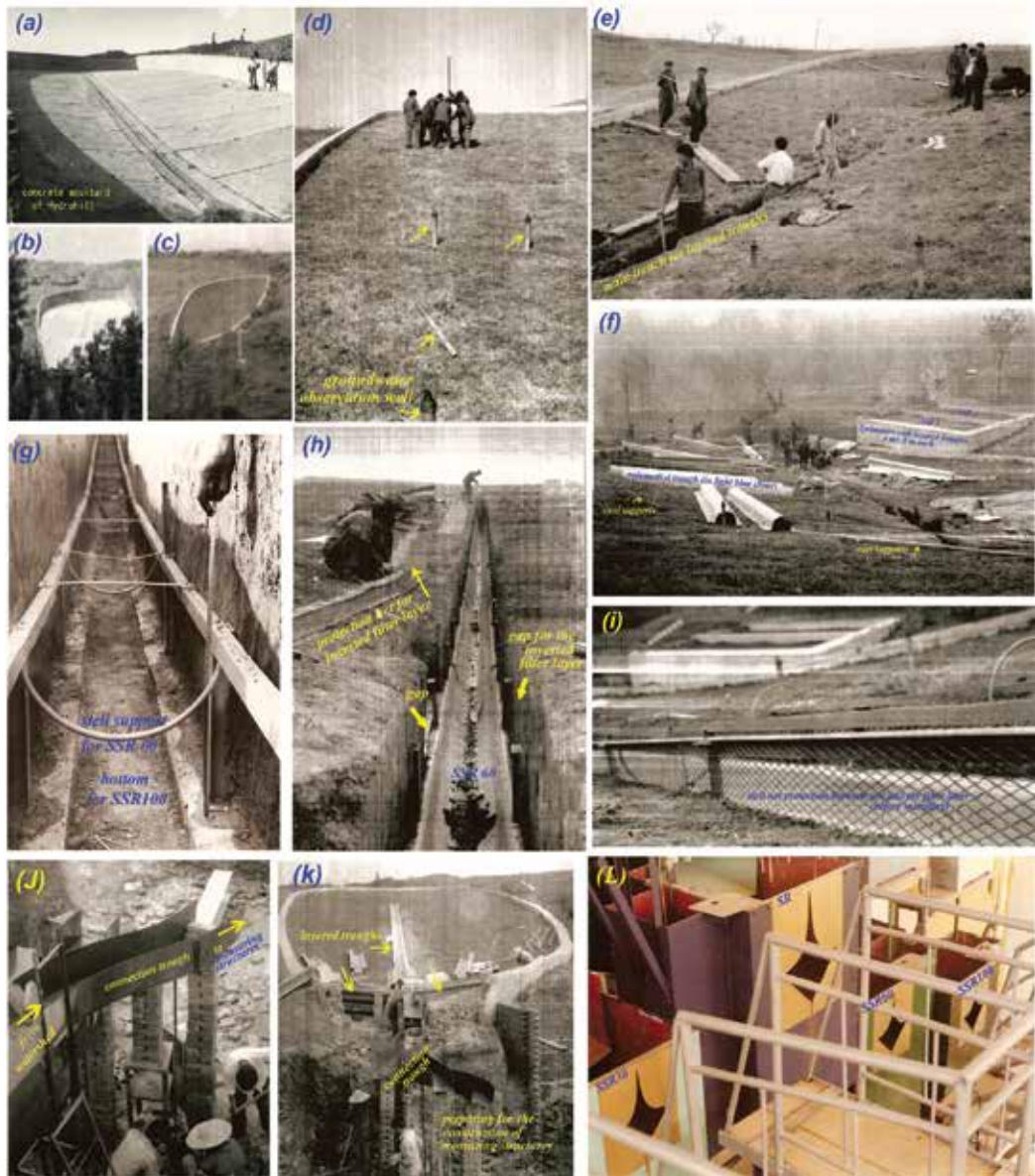
Figure 9. Constructions of Hydrohill. (a) the artificial aquiclude and surrounding wall; (b) view of the completed concrete aquiclude and wall; (c) view of the artificial catchment while soil was filled up, it was in idle for 3 years waiting for the physical improving of filling soil; (d) setting up monitoring networks for both saturated and unsaturated zone; (e) set drainage trenches; (f) the splicing fiberglass troughs and some steel supports; (g) the rectangular bottom trough for SSR100 and steel supports for the setting of SSR60 trough above it; (h) the gap for inverted filter and the nylon net in preparing; (i) the stainless steel screen in preparation for setting; (j) a curved connection trough; (k) connection troughs in installing; (l) discharge measuring structures using V-notch based logarithm sharp crested weirs (1982–1995).
