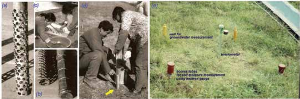
Figure 10. Construction of groundwater monitoring well. (a) the slotted part of steel tube; (b) the tube was wrapped up by plastic net; (c) making clay balls for using; (d) during installing, the space between the tube and drilling hole above the slotted lengths (shown by a yellow arrow) should be carefully stuffed up by small dried clay balls using a special designed tool. This picture is shown in commemoration of the late prof. M-Q Lu (left) of Nanjing University for his efforts and contributions. (e) a part of resulted networks showing well for groundwater, access tube for neutron moisture well and the tensiometer with connection plastic tubes to the scanner.
