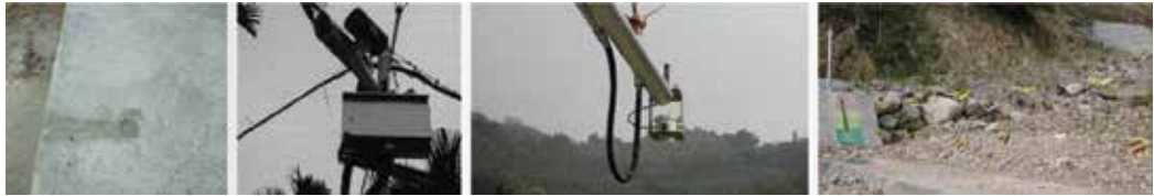
Figure 16. The equipment at the Shang'an Debris Flow Monitoring Sstation includes one rain gauge, one CCD camera, one geophone, two wire sensors and one water-level meter.
