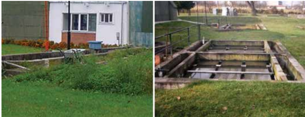
Figure 6. Inlet structure and efficient settlement tank on the WWTP Sokobanja.
