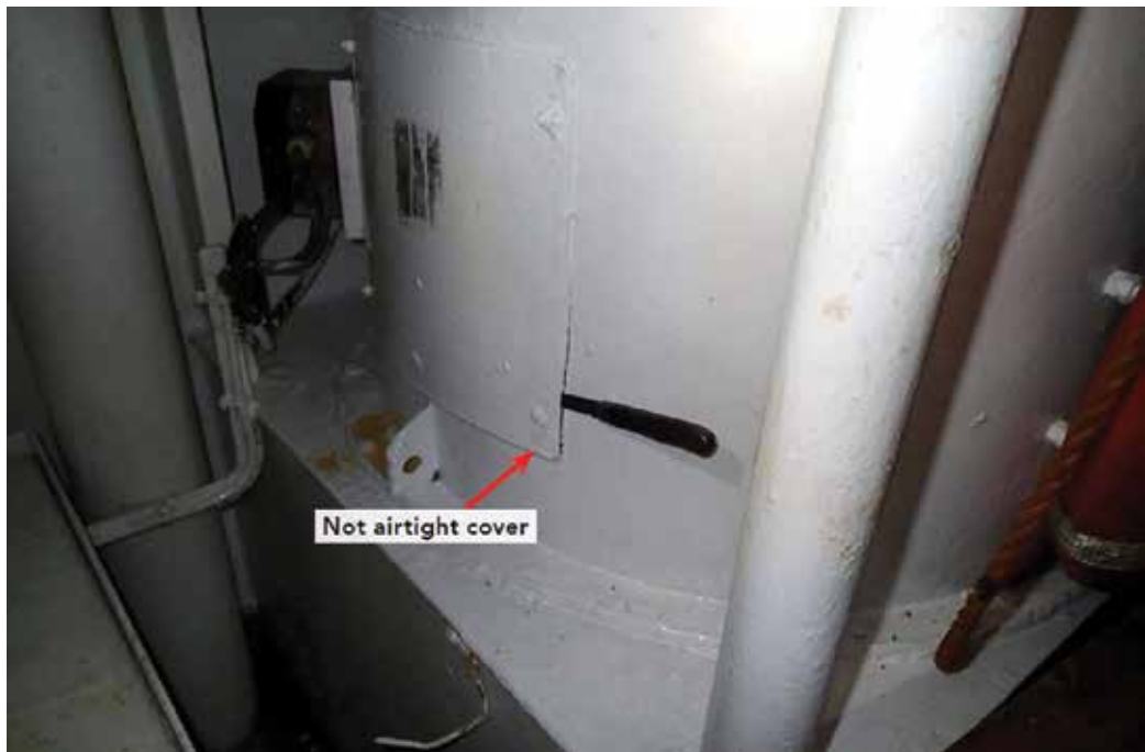
Figure 2. The inspection hatch on a ventilation duct that ran from the cargo hold through the forecastle. A minor gap in a section of the rim (knife blade inserted) allowed gasses to travel from the cargo hold to the bow area. (LADY IRINA). Source: [13].
