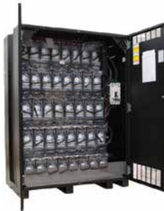
Figure 7. The batteries used to store generated energy.
