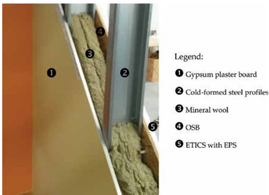
Figure 2. Materials in a LSF wall crosssection [30]. Legend: Gypsum plaster board; Cold-formed steel profiles; Mineral wool; OSB; and ETICS with EPS.
