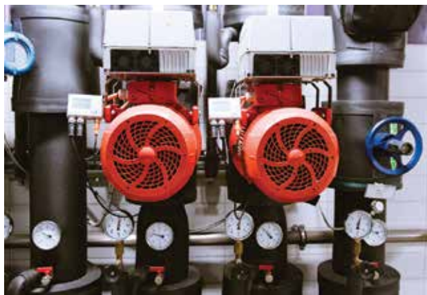
Figure 10. Geothermal loop system hole connections with valves.
