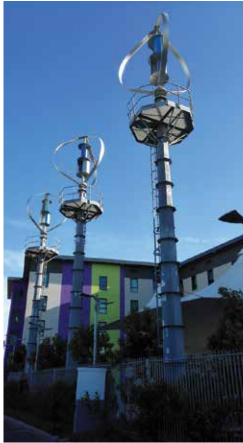
Figure 4. Huebner-Giessen 3 kW wind turbines.
