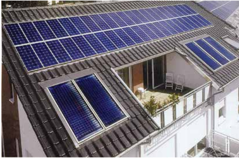
Figure 17. Photovoltaic panels integrated into building [49].
