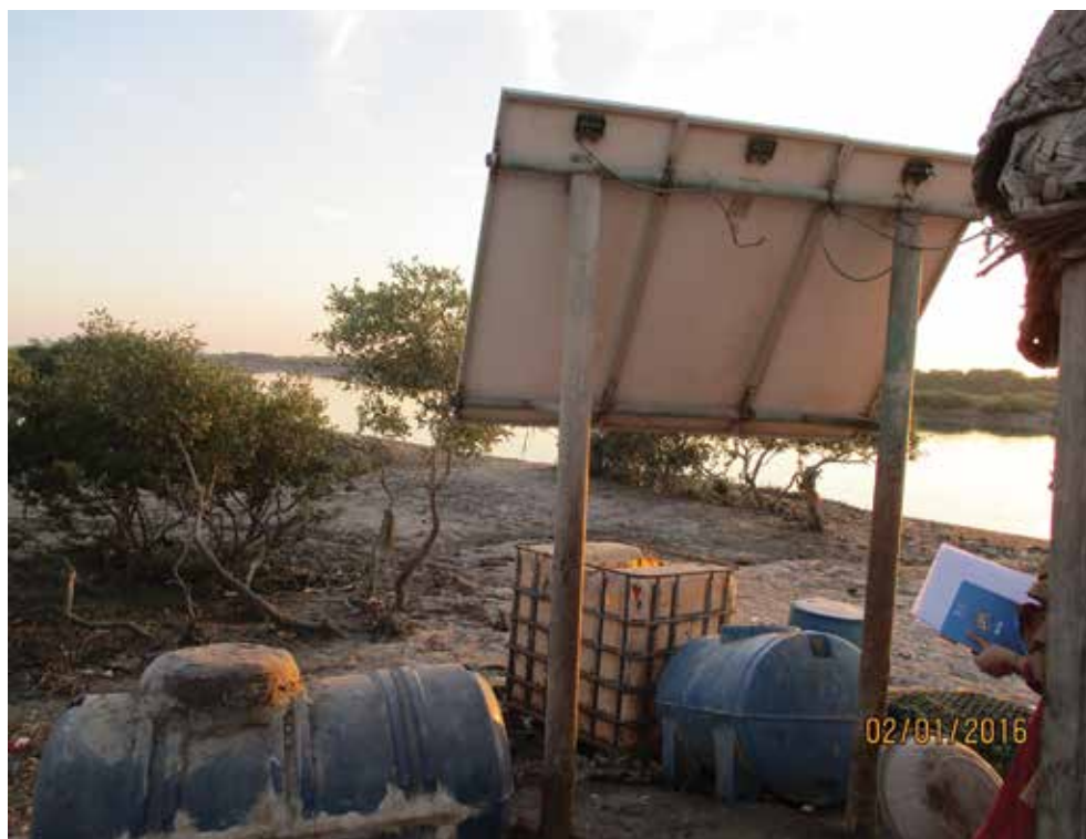
Figure 9. Broken solar panels require maintenance and repairs; the only source of power to recharge torch and mobile phone batteries.
