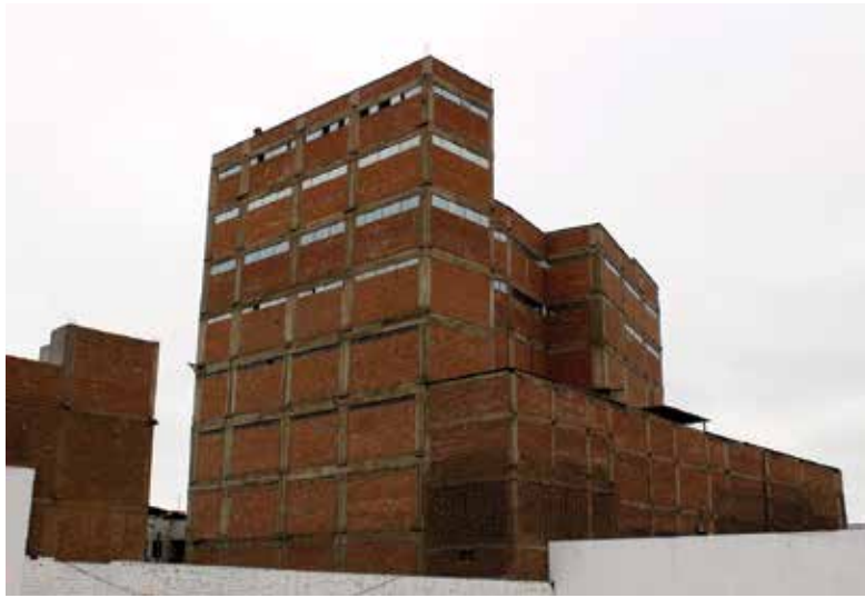
Figure 2. The storage facilities that violate the building height restrictions for the historic centre and come to replace the old structures within an area deemed of monumental value. Source: Photo by Rita Lambert.
