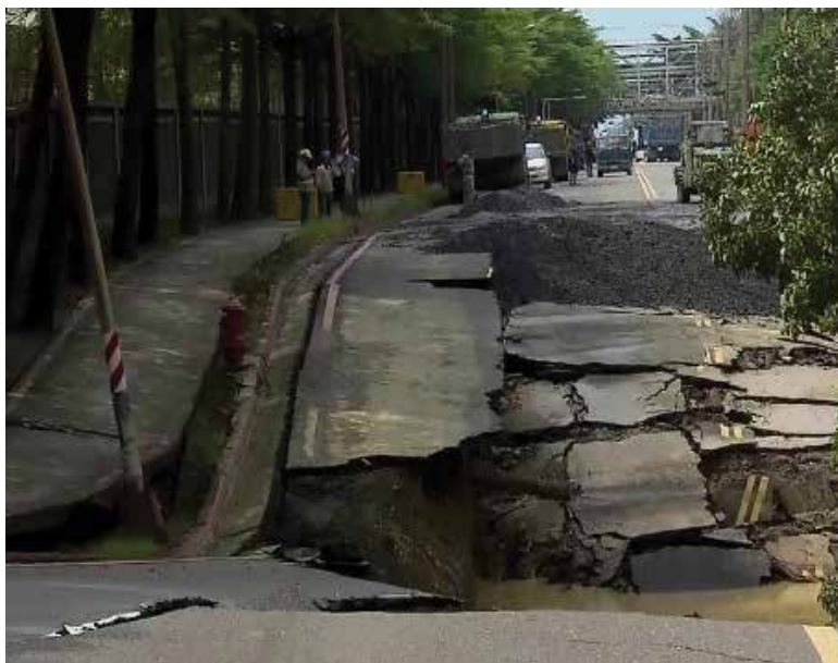
Figure 2. Destruction of roadway.
