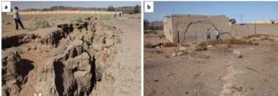
Figure 3. Photographic pictures showing (a) Earth fissures' distribution, (b) Impact of earth fissures on buildings.
