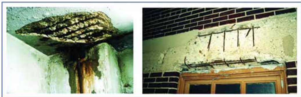
Figure 2. Deterioration of normal concrete [7].
