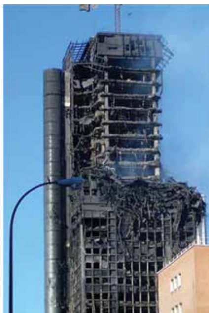
Figure 1. Damage of concrete and reinforcement after Madrid Windsor Tower fire (Spain, 2005).
