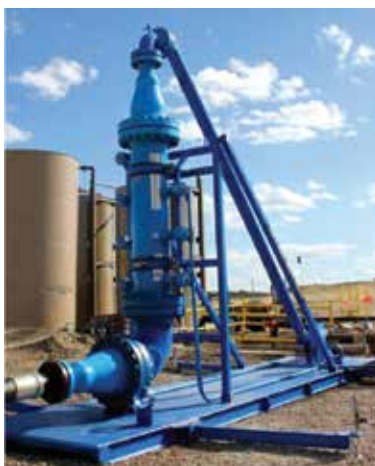
Figure 9. The photo of the AOT device installed in the pipeline.
