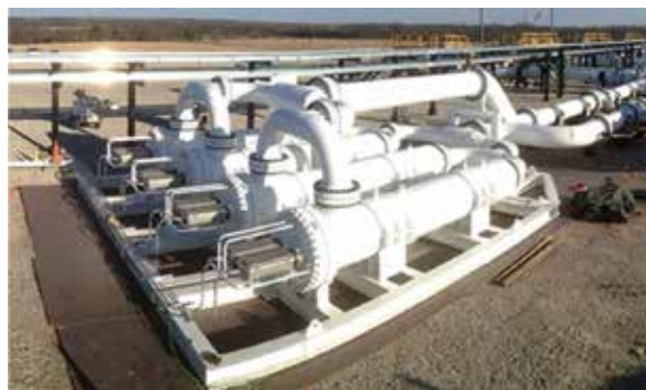
Figure 12. AOT device installed on the Keystone pipeline system.
