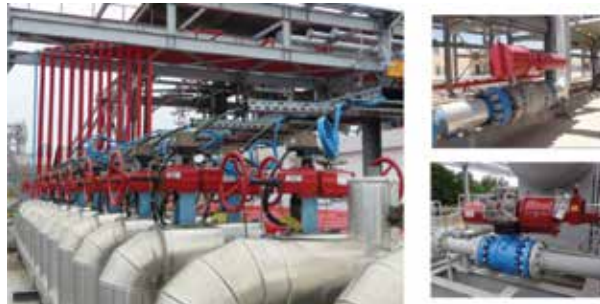
Figure 7. Example of emergency shutdown valve.
