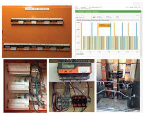
Figure 7. Installed Embedded Network Installations in 2015 at Murdoch University: from top left and left to right each row (a) 9x SATEC EM133 meters installed on main distribution board in one building, (b) chart showing output from the Schneider Electric COM510 energy server webpage, (c) showing the 3x energy servers with ethernet and modbus connections, (d) and (e) showing the EM133 smart meter installation using IPD CTs, test links and voltage fuses.
