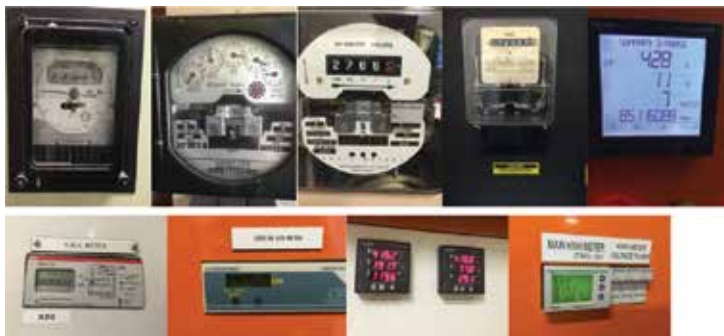
Figure 6. The variety of existing meters installed at Murdoch University.
