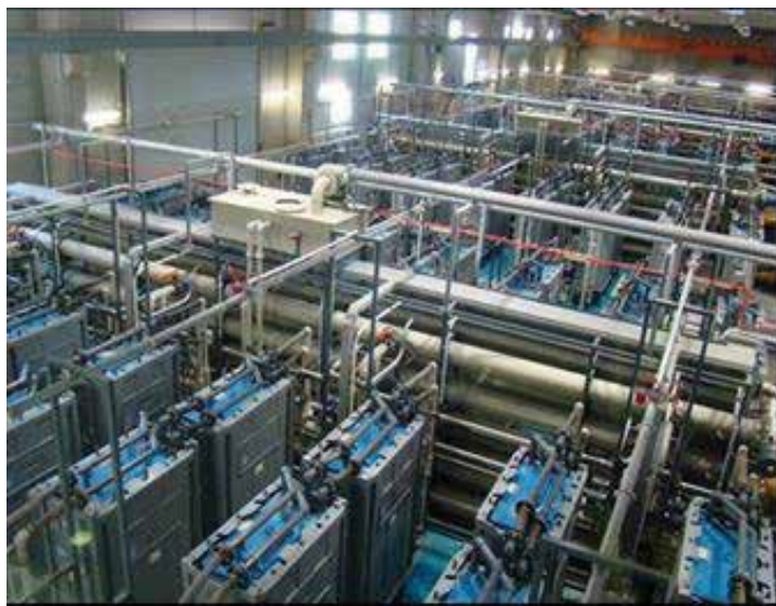
Fig. 3. Details of the EDR step at the Abrera DWTP.
