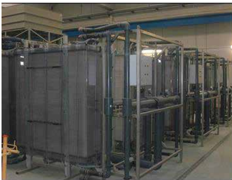
Fig. 4. EDR stacks at the Depurbaix WWTP.
