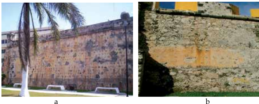
Fig. 2. General aspect of degradation at Forts San Pedro (a) and San Carlos (b), historic buildings of San Francisco de Campeche City.
