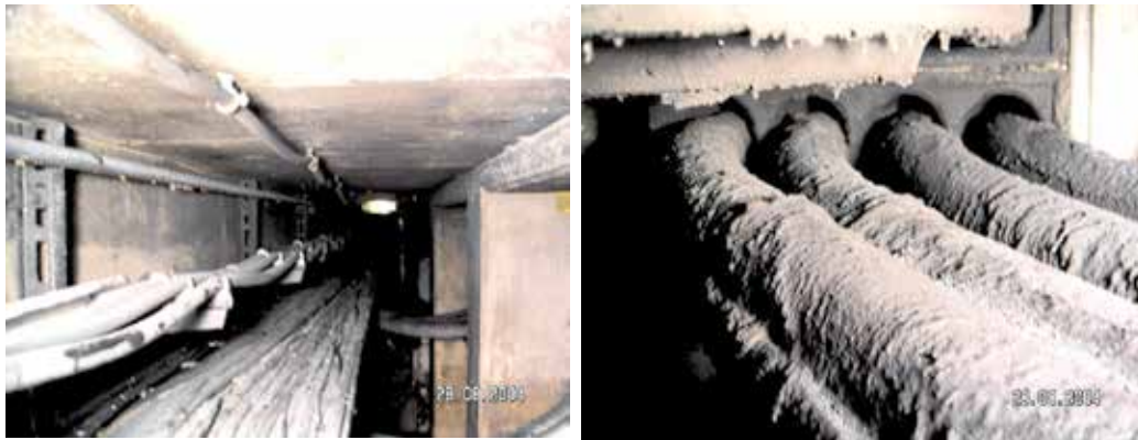
Fig. 4. Cables with protection by intumescent coating; left: photo of the cable channel, right: photo of the coating
