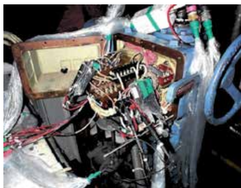
Fig. 2. A picture of installed sensors at a valve test
