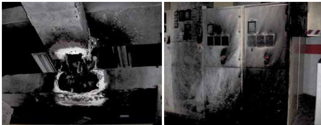
Fig. 9. Photographs of the damages at the Diablo Canyon nuclear power plant (from Brown et al., 2009)
