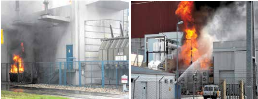
Fig. 8. Flame and smoke occurring at the generator transformer; the photo on the right hand shows the fire extinguishing activities
