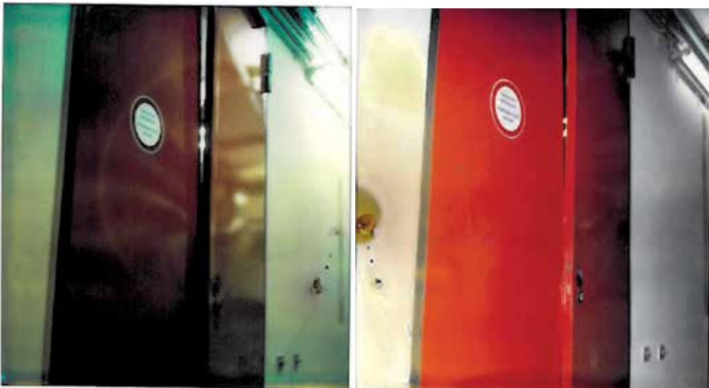
Fig. 6. Photographs of the damaged fire door from outside the room
