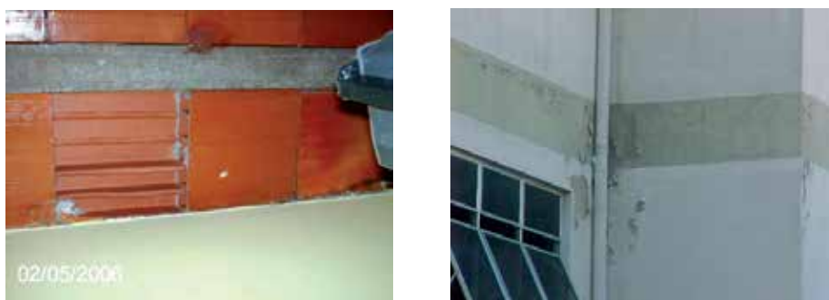
Fig. 3. Detachment of the floor brick and walls
