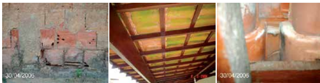
Fig. 1. Fast degradation of masonry and tiles
