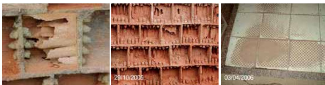
Fig. 4. Fast degradation in masonry due to saline spray and abrasion
