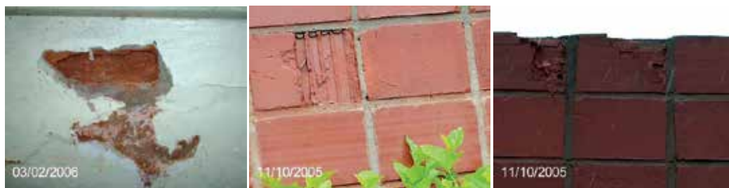
Fig. 2. Fast degradation of masonry due to sulfate water and temperature change
