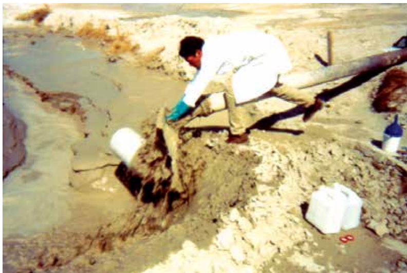
Fig. 1. Pipe used to transport the solid residuals until the jales dam
