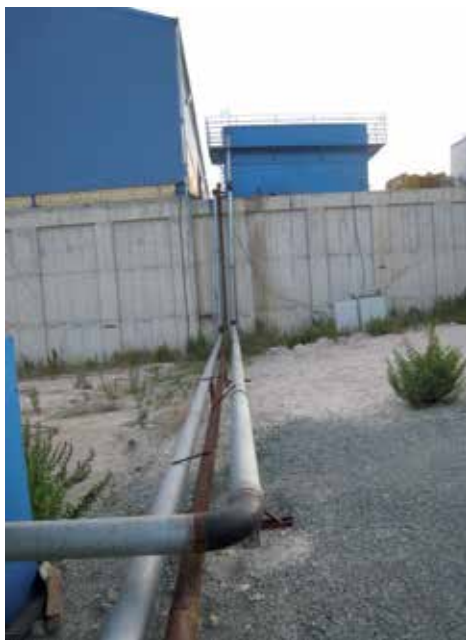
Figure 12. Constant head tank, connection to the experimental network
