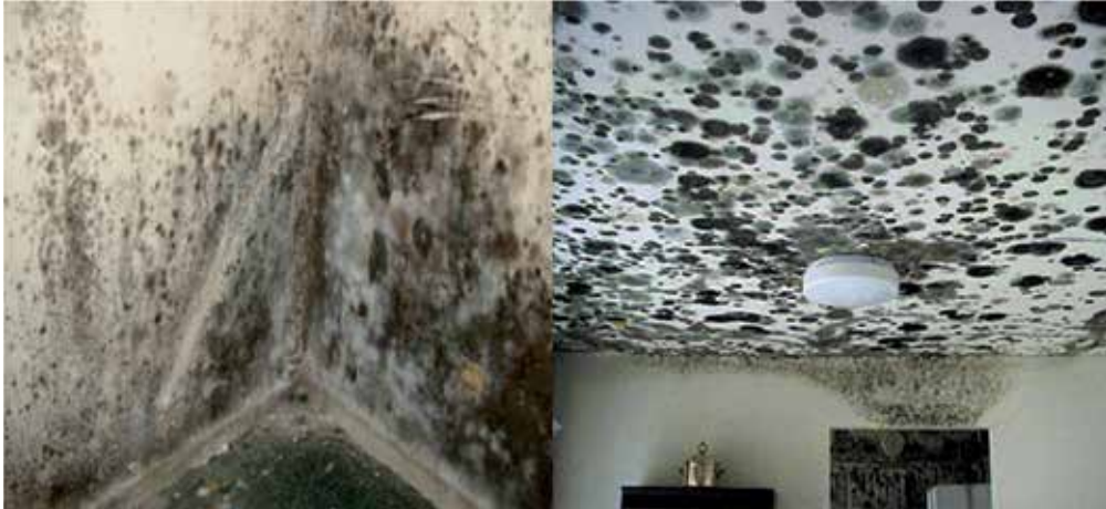
Plate 2. Fungi on the wall and ceiling of a typical indoor environment
