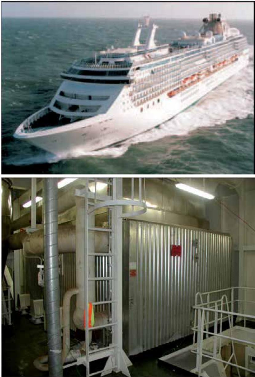
Figure 10. Coral Princess at sea and boiler installed on ship [63]
