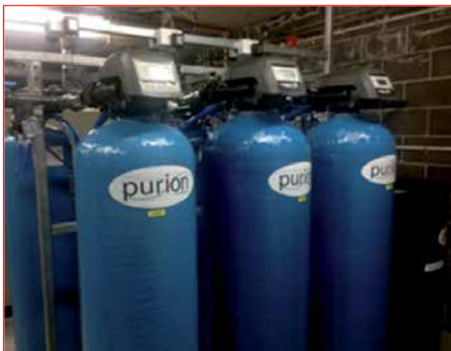
(A) 2 carbon filters, 1 softener tank and a brine tank in series.
