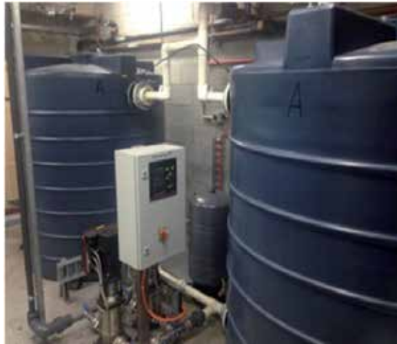
A) Two 3000L holding tanks to provide an uninterrupted water supply in case of emergency. Note also the booster pumps in the centre. These ensure an inlet pressure of at least 550Kpa
