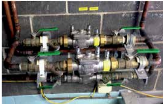
(B) A backflow device.
