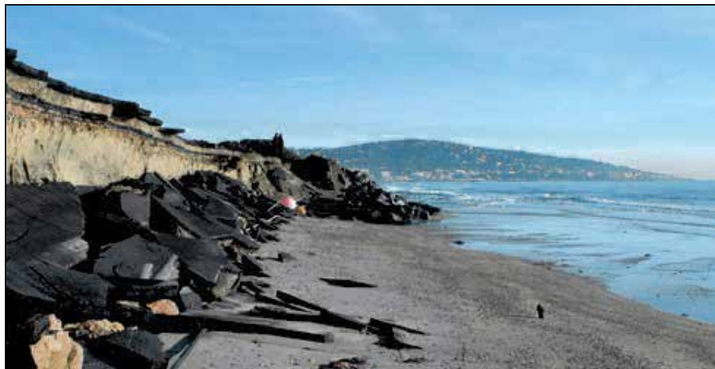
Fig. 12. Frequent destruction of coastal road due to storms (source DREAL LR)
